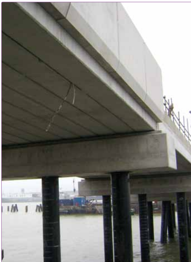
Cementitious coatings can also be used to enhance cover on new construction, such as the link bridge at Belvedere Riverside Energy from Waste (EFW) facility in South East London
