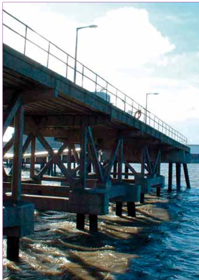
Cementitious Coating 851 was specified for application to supporting pillars of a jetty in the North West of England
