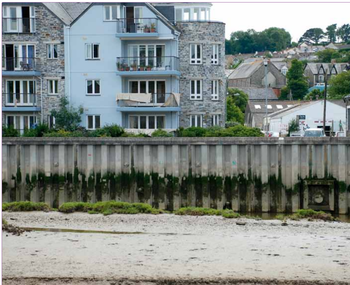
As well as protecting reinforced concrete, cementitious coatings are also ideal for the corrosion protection of steel, as demonstrated by a project at Wadebridge Estuary in Cornwall where the steel sheet piling was protected
