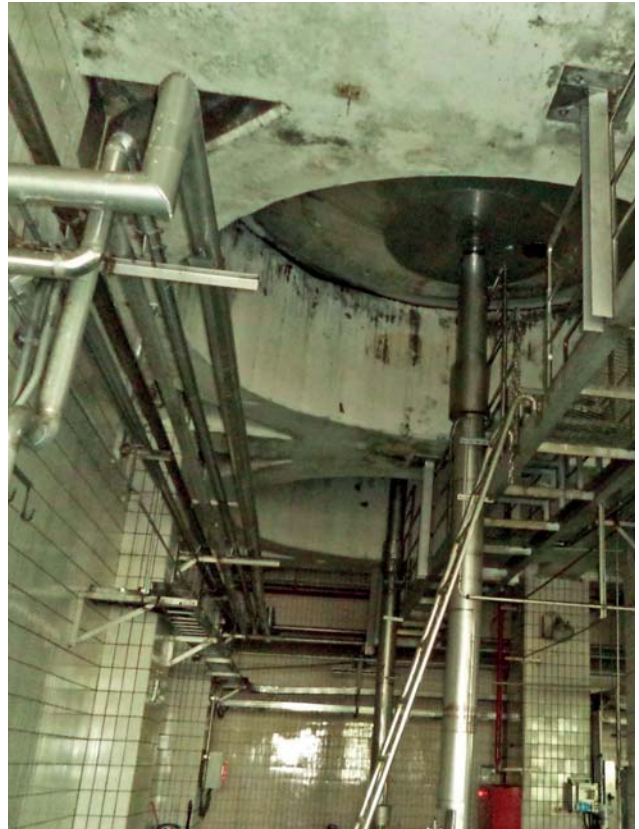
Above and below left: Problems with mould growth before the application.
